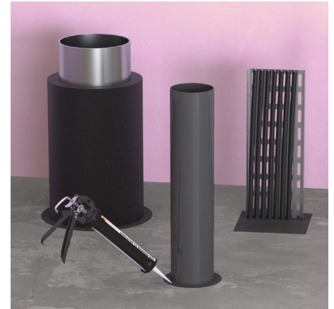
QuelStop HPE Sealant used around service penetrations through floors
